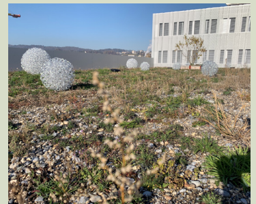
Extensive green roofs are very rich from an ecological point of view, both for fauna and flora.
